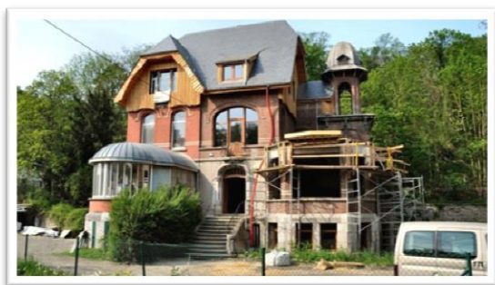
Saint-Servais © Christian Delwiche
